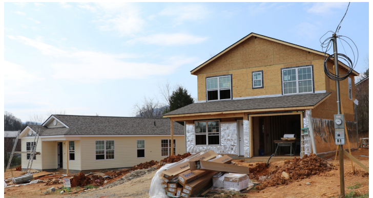
Houses under construction in the Tri-Cities that fit the affordability range for families who will benefit from Project Reinvest.
